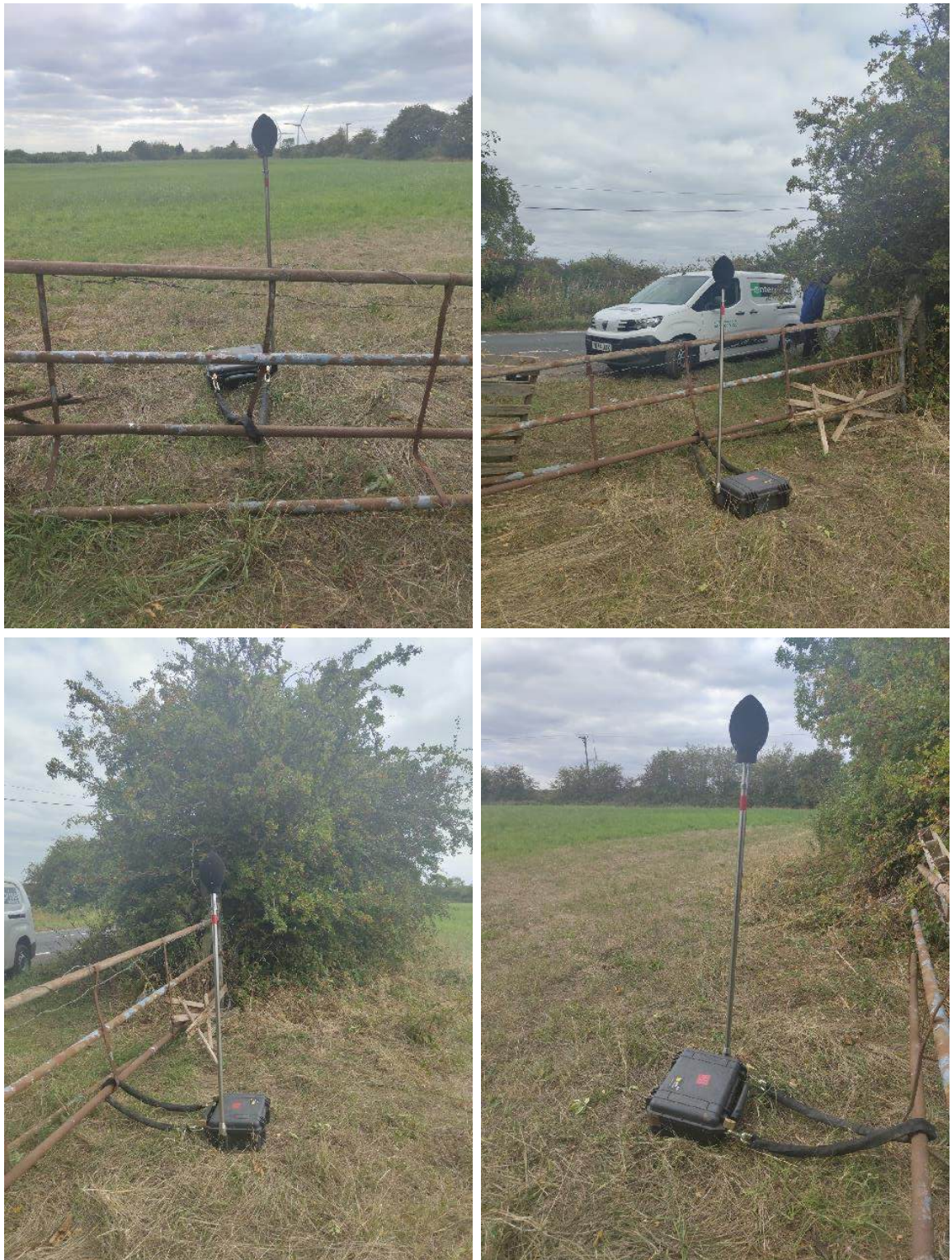
Figure 14.2-25: Photos of Equipment at NML11
