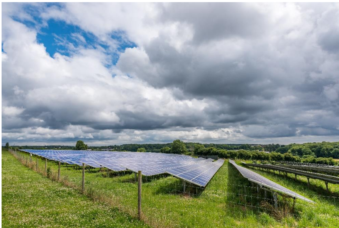
Image 1: Typical example of solar PV array
