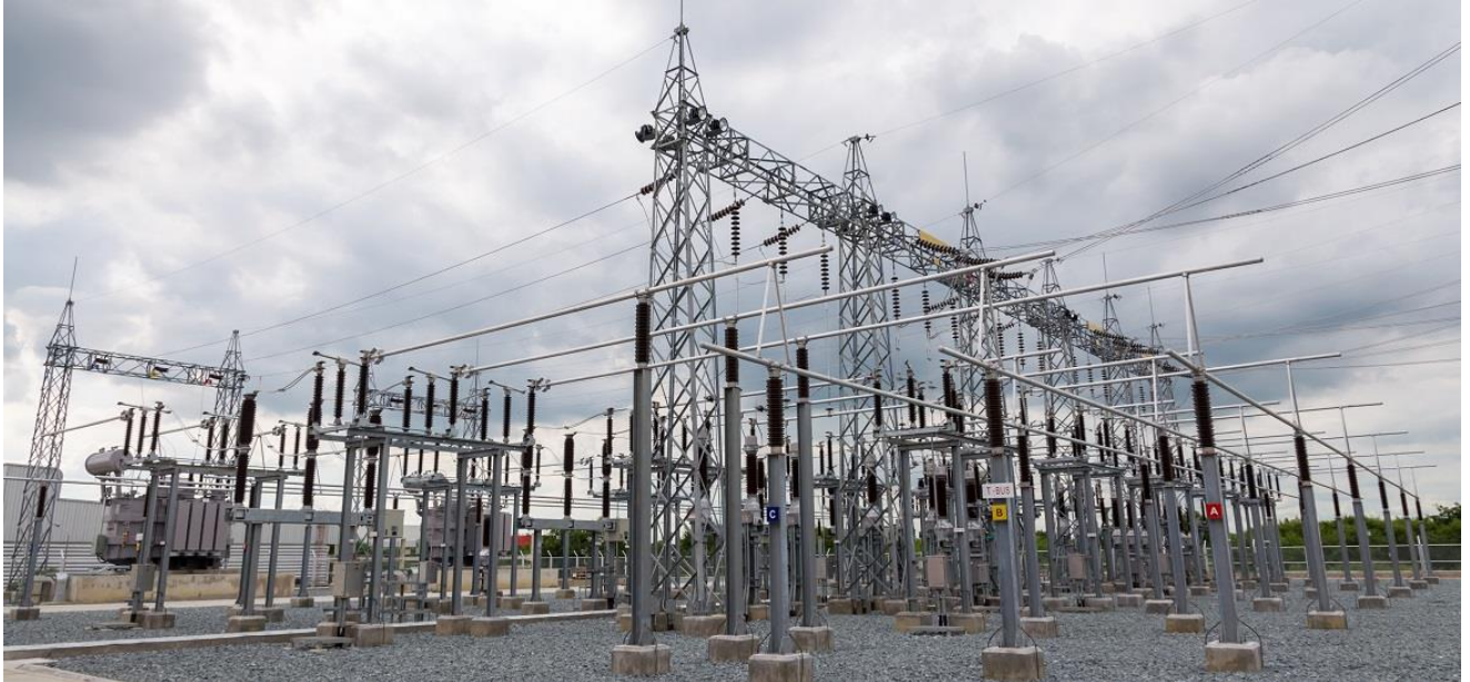
Image 4: Example of a 400kV substation
