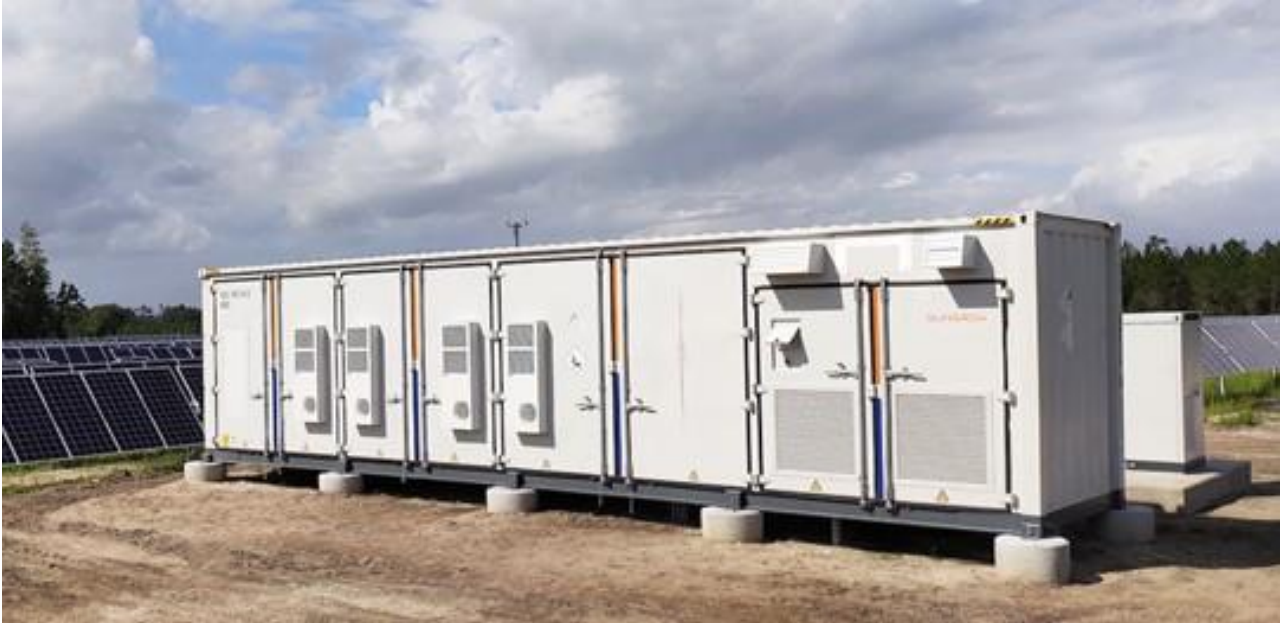
Image 3: Example of a BESS unit
